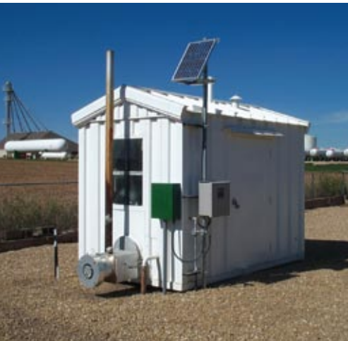
Location: Central Iowa System Size: 40 W
